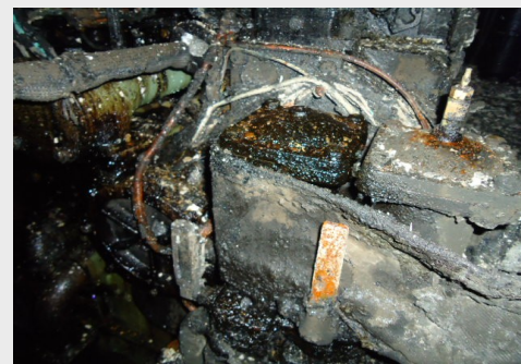
Figure 2: Fuel filters of No.3 Generator
